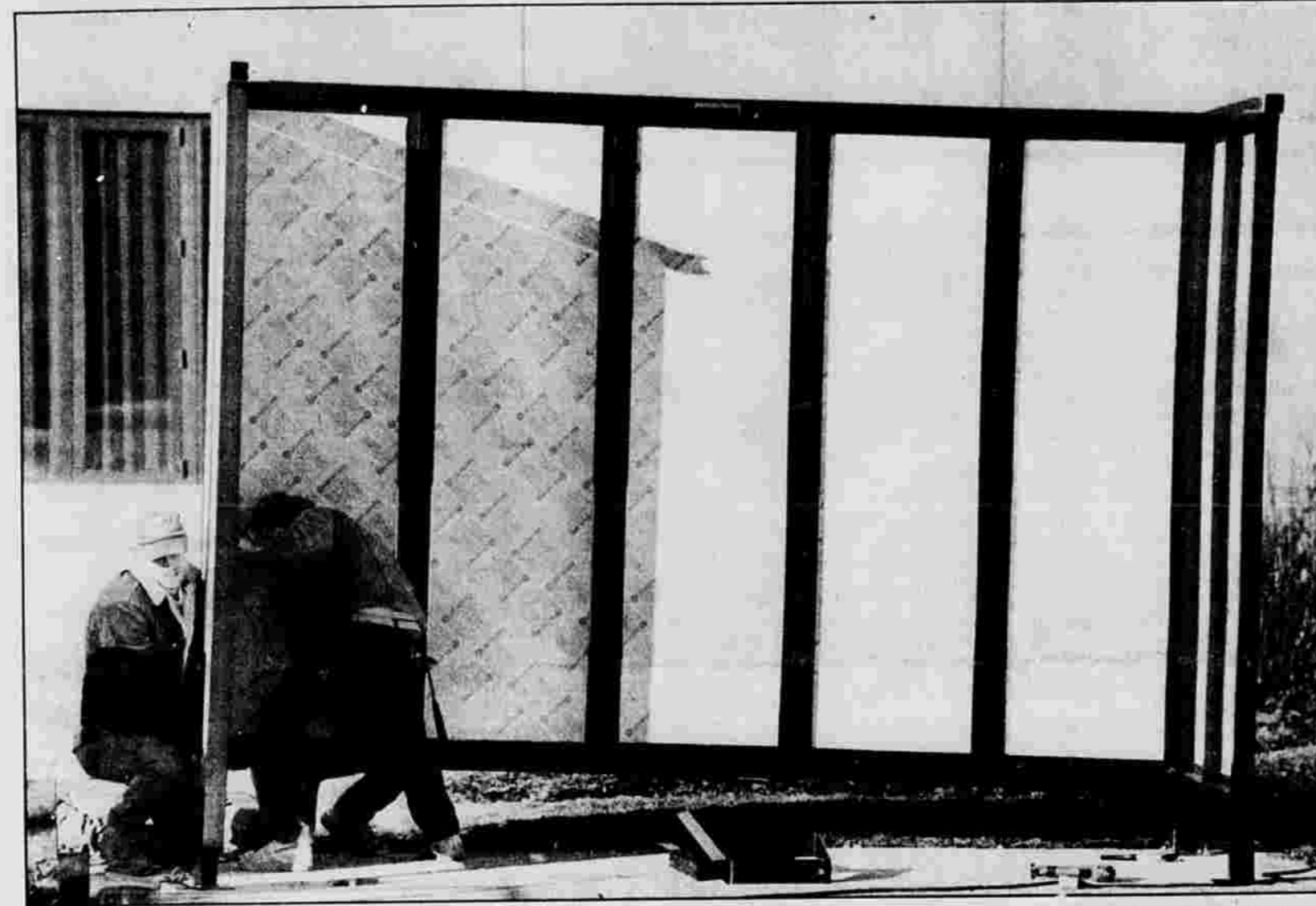
SHELTER — Mark Marden of Chaplin, left, and Jeff Guibeault of Willimantic put up a bus shelter at Manchester Community College today. The two carpenters, who work for DmC Construction Co. of Manchester, estimated it would take about two hours to complete their work.
